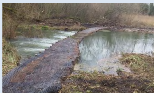
Fig 3b: Main weir on Middle Ditch, Jan'16, showing completed weir with previously eroded by-pass channel in the foreground (looking across channel)
