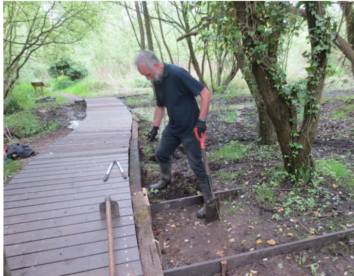
Using old railway sleepers and other boards to make bunds to retain water along margin of new boardwalk, 21.05.2016.
