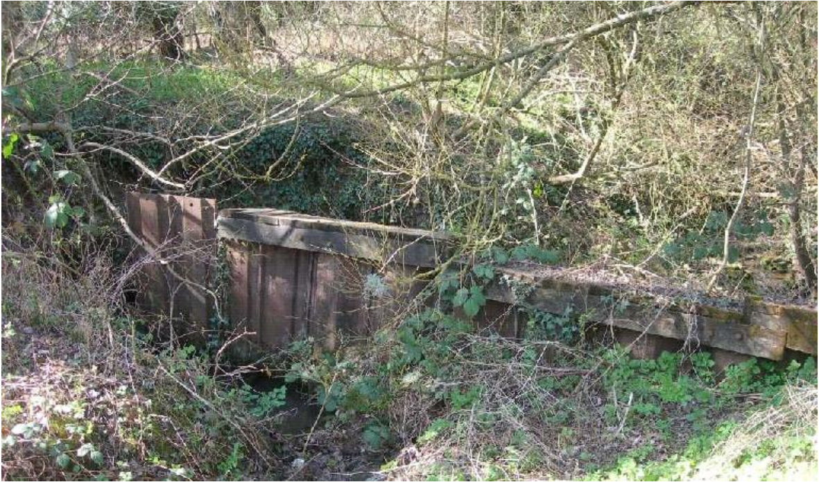
Metal and wooden structure that previously formed a barrier across the stream, now non-functional due to bank erosion around one end
